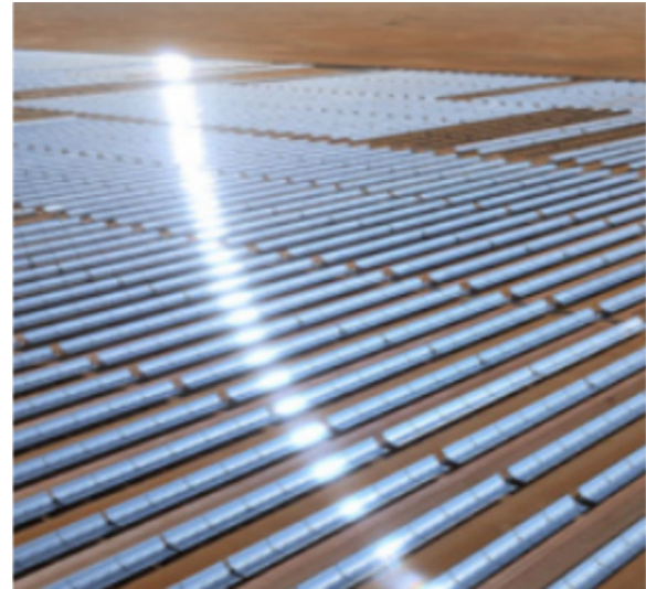
Fig. 6 Solar farms to generate electrical energy in Masdar city 2019 (Source: Annual Report 2022)
